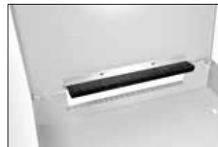
Zone Cabling Enclosure hinged open.
