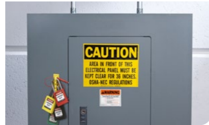
Panel and Enclosure ID
