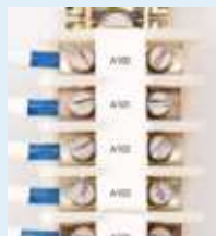
Terminal block marking
