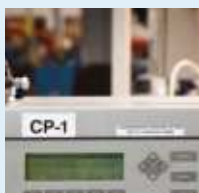
Control panel and electrical panel labels
