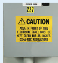
Hazard warning signs
